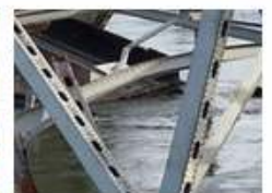
I-5 bridge collapses in northwest Washington
